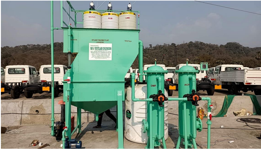
Sewage Treatment Plant, Rudrapur Stockyard
