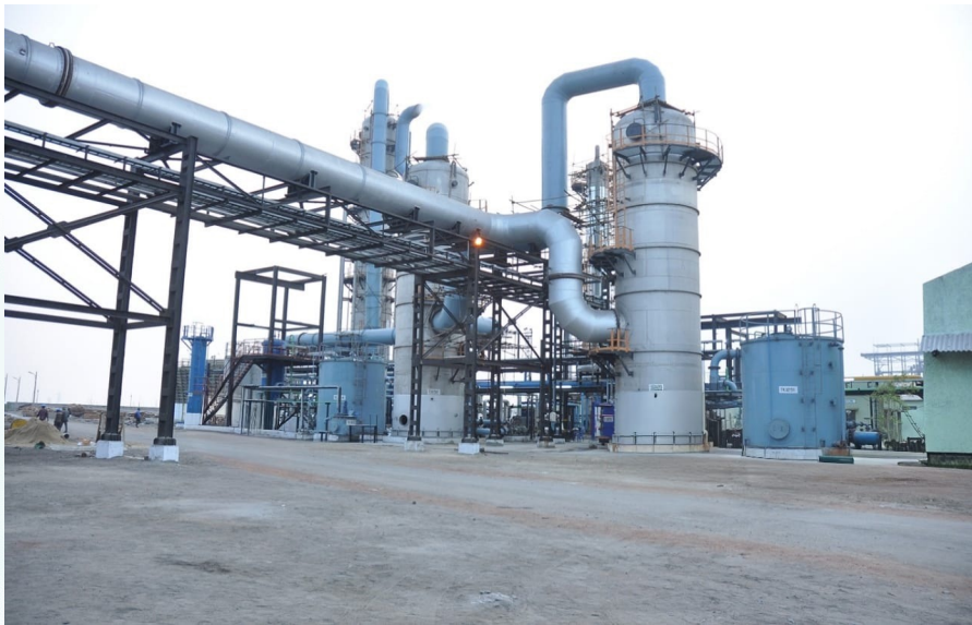
174MTPD CARBON CAPTURE PLANT
