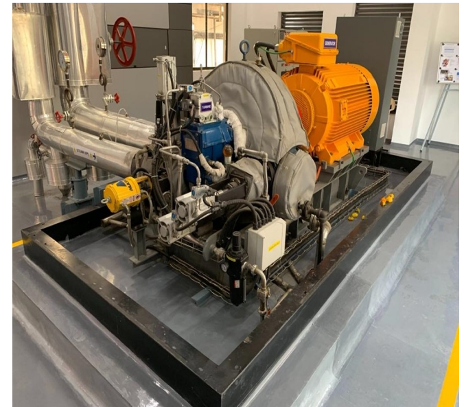
Energy recovery through 700 KVA IG turbine
