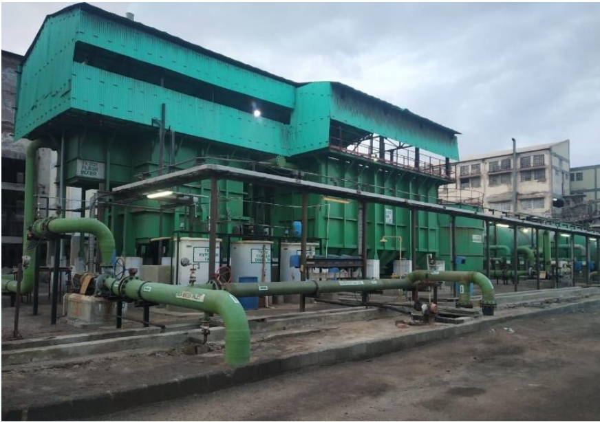
3MLD DESALINATION PLANT
