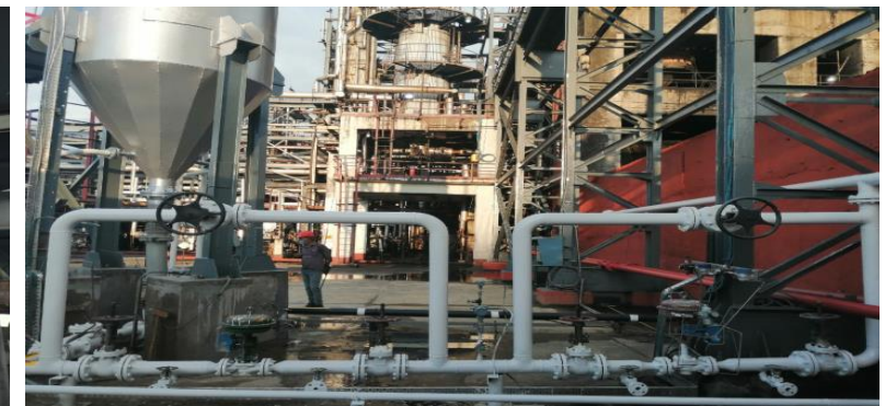
Conveying gas line
